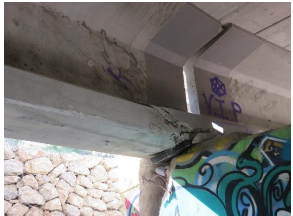
Figure 5. Damaged precast beam. Note the state of the neoprene bearing pad.
