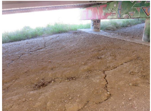
Figure 4. Tension cracks on the soil surface below the bridge
