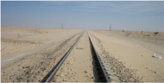
Figure 2 Blowing sand on NSR Project Segment 7 close to Al Jubail area
