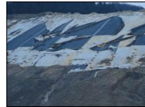
Figure 3. Example 3 – closing of an old landfill – improper design of the side slopes without geotechnical calculations
