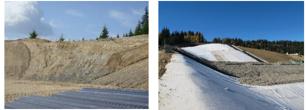
Figure 2. Example 2 – new landfill – improper design of the side slopes without geotechnical calculations – before (left) and after remodelling (right)
