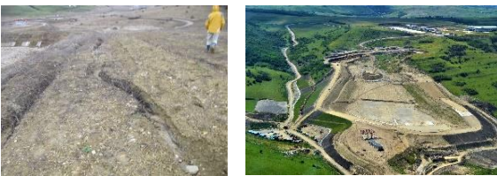
Figure 6. Example 4 – new landfill – improper design and execution of the dikes (left), after reconstruction (right)
