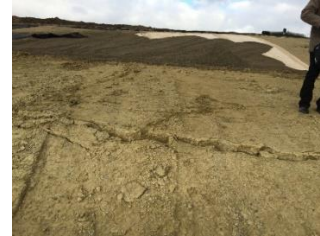
Figure 9. Case study – old landfill – fissures appeared during the capping works – slope
