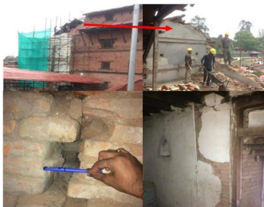
Figure 10 View of the collapsed portion of the courtyard building
