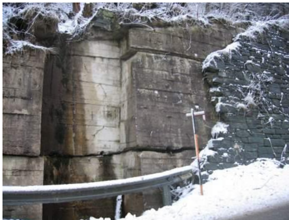
Figure 9. Damage to retaining walls along "old" route
