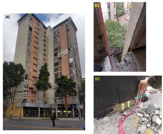
Figure 2. The Osa Mayor rocking failure: (a) plan view of the 15-floor RC double L-shaped building, (b) the opening between the two L-buildings as seen from the 11 th floor, and (c) detail of the uplifted corner (with the turquoise double end arrow is noted the horizontal gap induced by the rocking motion of the building).
