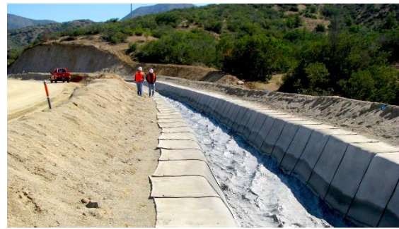
Figure 3. Use of a GCCM to line a tailings ditch carrying liquid made up of up to 60% solids
