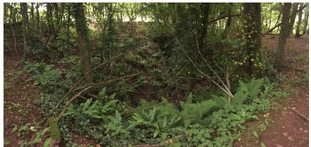
Figure 3 Surface depression at Pembroke Tunnel with mature trees growing within.
