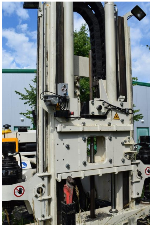
Figure 2. DP machine pushes the CPT based seismic tomographic system into the ground
