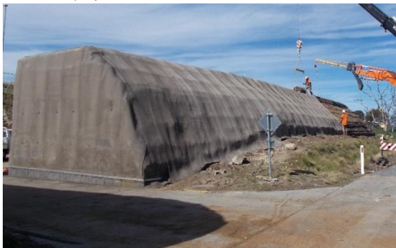
Figure 9. Installed GCCM to protect wrap faced bund. Courtesy of Concrete Canvas Ltd.
