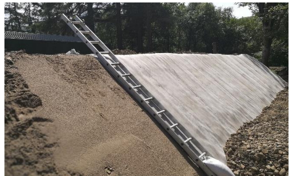
Figure 11. Sand placed on face of RSS prior to placing GCCM. Courtesy of Concrete Canvas Ltd.
