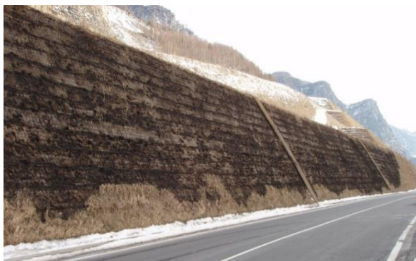
Figure 7 The reinforced structure after the fire event
