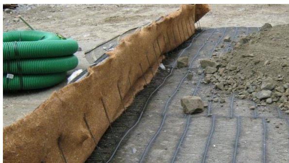
Figure 5 Installation: from the left, steel mesh formwork, geogrid, straw mat, and fill material.
