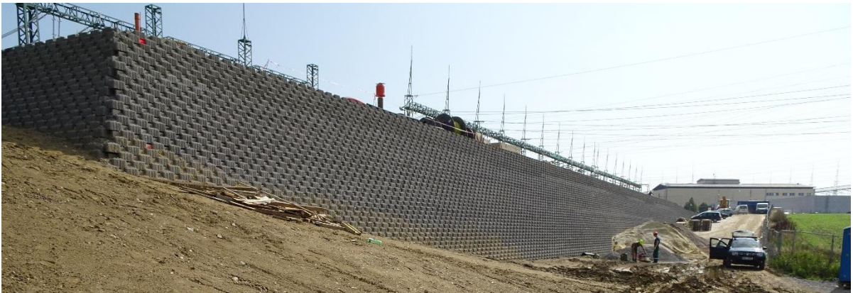
Figure 9: Finished reinforced soil retaining wall with small concrete facing blocks and slope of 66^\circ , view of maximum height section
